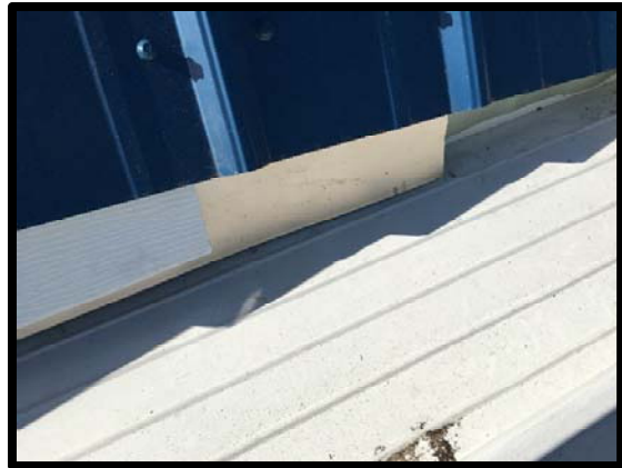
Picture 2: Limited or no flashing
