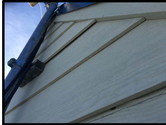
Picture 10: Loose Hardi plank siding
