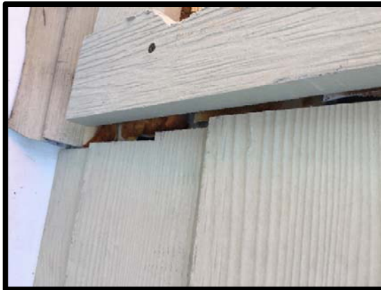
Picture 11: Limited or no Tyvex and caulking at gaps
