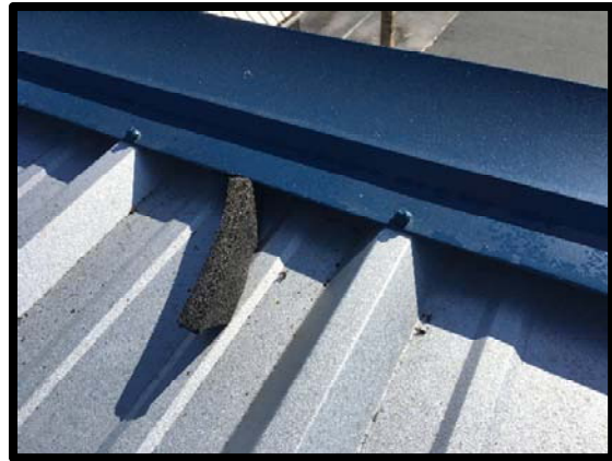
Picture 8: Loose foam beneath roof cap
