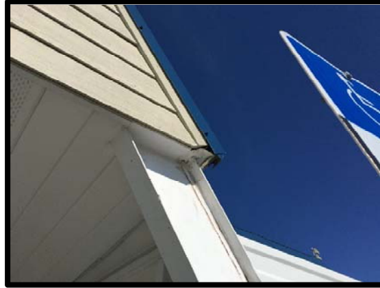
Picture 12: Gap at roof and gable edges
