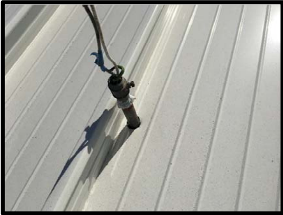
Picture 1: Penetration with no caulking
