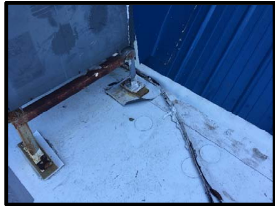
Picture 4: AC Unit on loose TPO section
