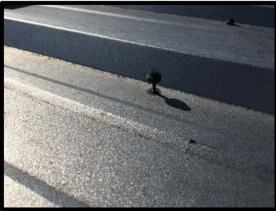
Picture 7: Loose roof screw
