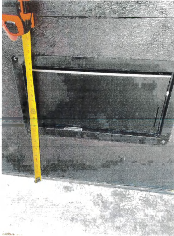
Garage door vent X 2 (only 1 photo)
