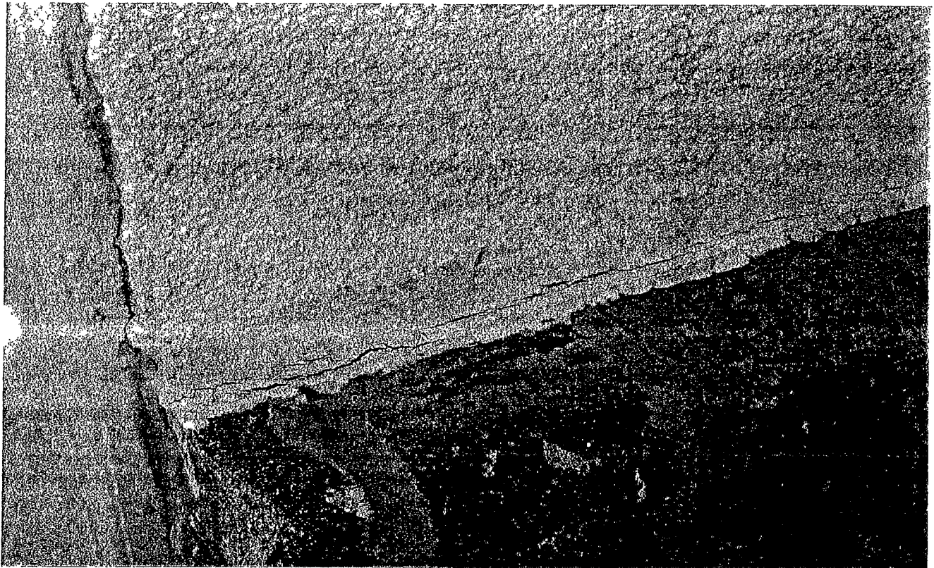
VIEW 11: HORIZONTAL CRACK - NORTH SIDE OF HOUSE - WEST OF EAST DOOR ENTRANCE
