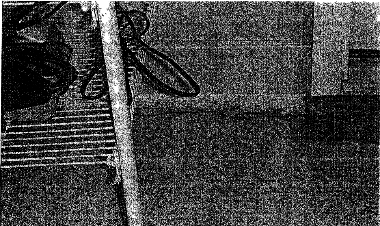
VIEW 44: SLAB SEPARATION - GARAGE - SOUTHWEST CORNER
