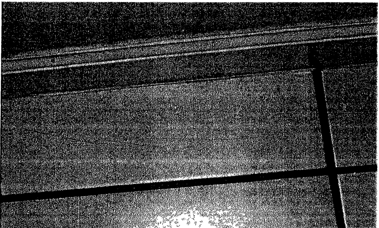
VIEW 50. TILE CRACK - KITCHEN - EAST END, NEAR HALLWAY ENTRANCE
