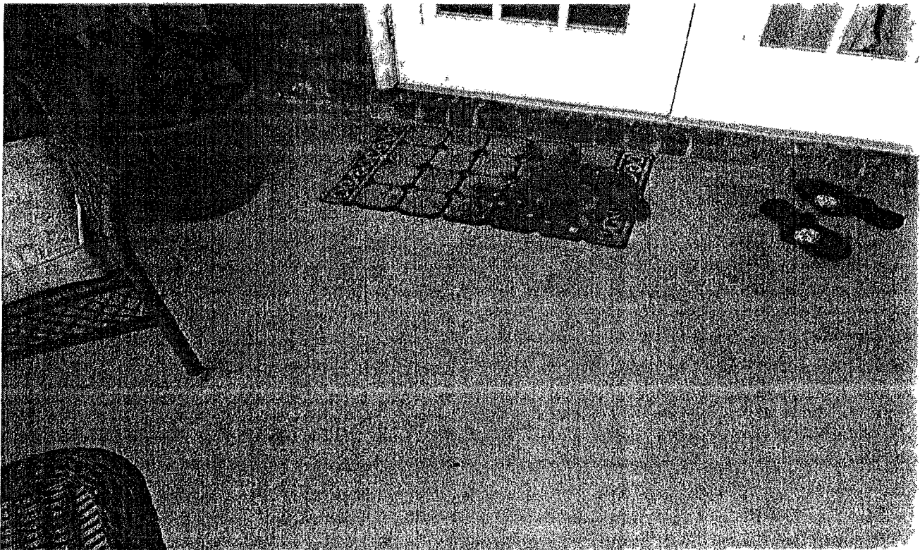
VIEW 18: SLAB CRACK - BACK OF HOUSE - BACK PORCH, NEAR NORTH FRENCH DOORS
