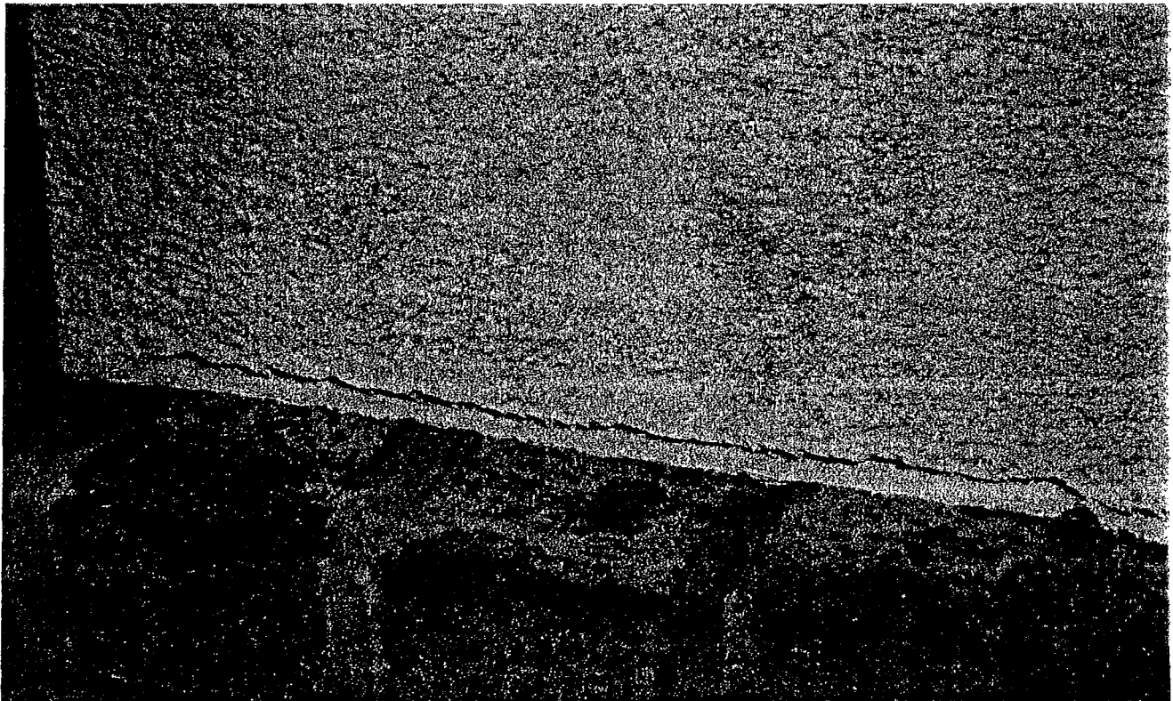
VIEW 42: HORIZONTAL CRACK - SOUTH SIDE OF HOUSE - SOUTHWEST CORNER
