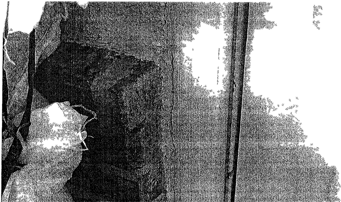
VIEW 10: DOOR TRIM SEPARATION - NORTH SIDE OF HOUSE - EAST DOOR ENTRANCE
