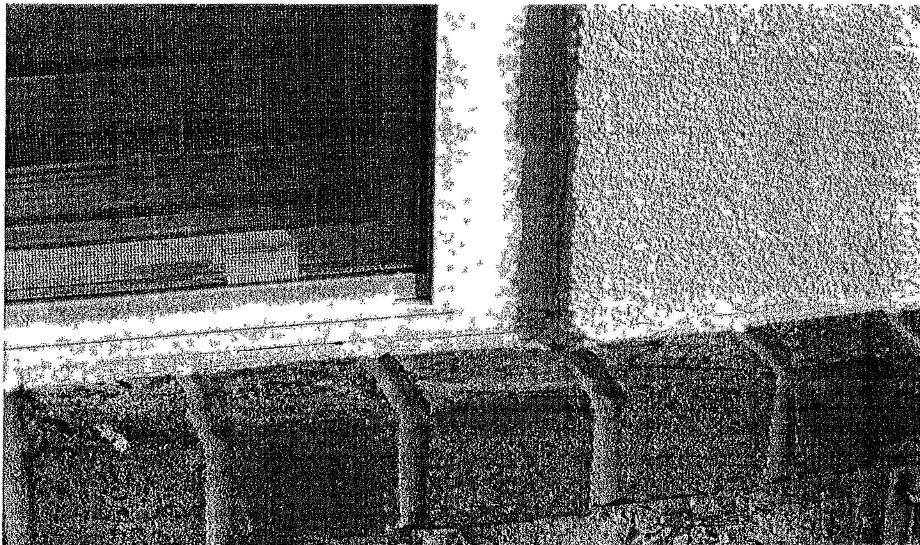
VIEW 30: WINDOW SEPARATION - FRONT OF HOUSE - NORTH WINDOW
