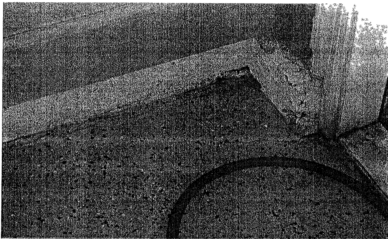
VIEW 47: SLAB CRACK - GARAGE - NORTHWEST CORNER
