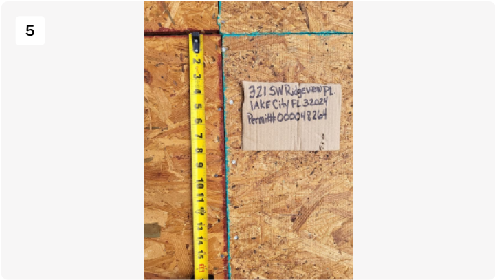
Project: Massey Date: 10/5/2023, 11:33am Creator: Sean Baucom
