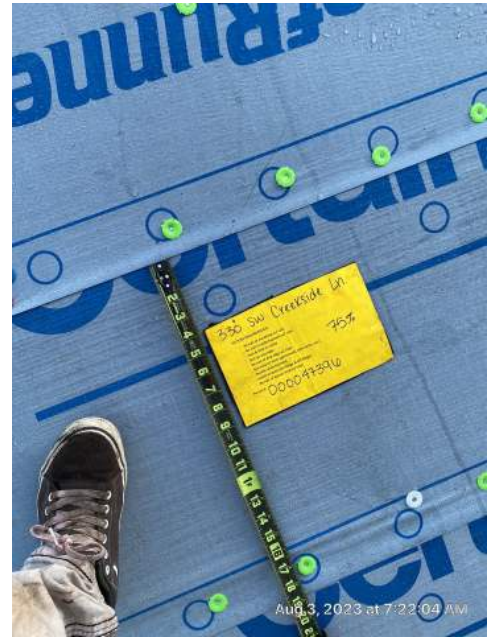
Carruthers 4781 330 SW Creekside Ln • Lake City, FL 32025 Thu, Aug 3 07:22 am by Terry Lewis
