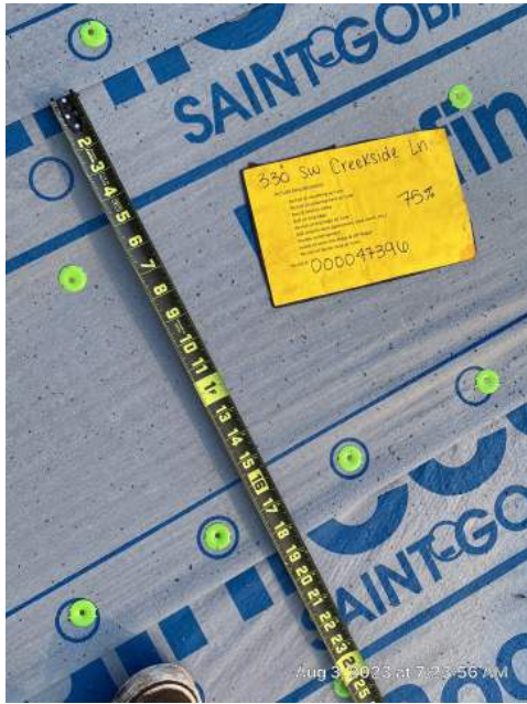
Carruthers 4781 330 SW Creekside Ln • Lake City, FL 32025 Thu, Aug 3 07:23 am by Terry Lewis
