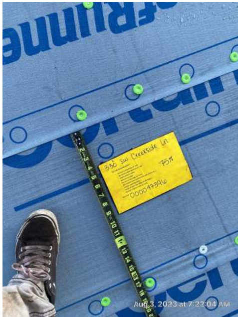
Carruthers 4781 330 SW Creekside Ln • Lake City, FL 32025 Thu, Aug 3 07:22 am by Terry Lewis
