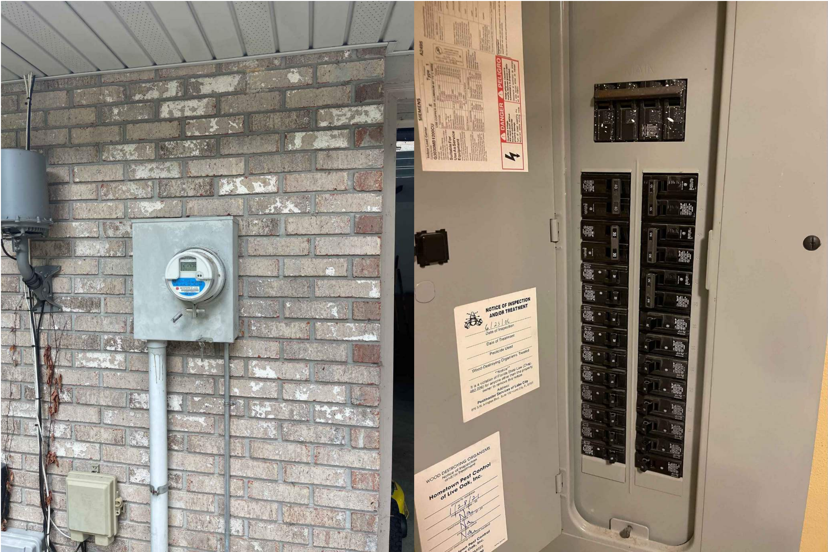
1 EQUIPMENT PHOTOS SCALE: NTS
