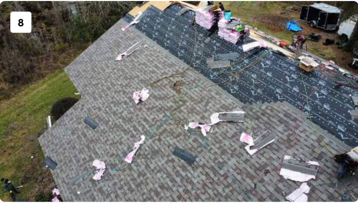
Project: Michael McKee #8170 Truss Repairs. Engineering in the file.. $1550 for engineering. Date: 1/24/2025, 3:19pm Creator: Thomas Grigsby
