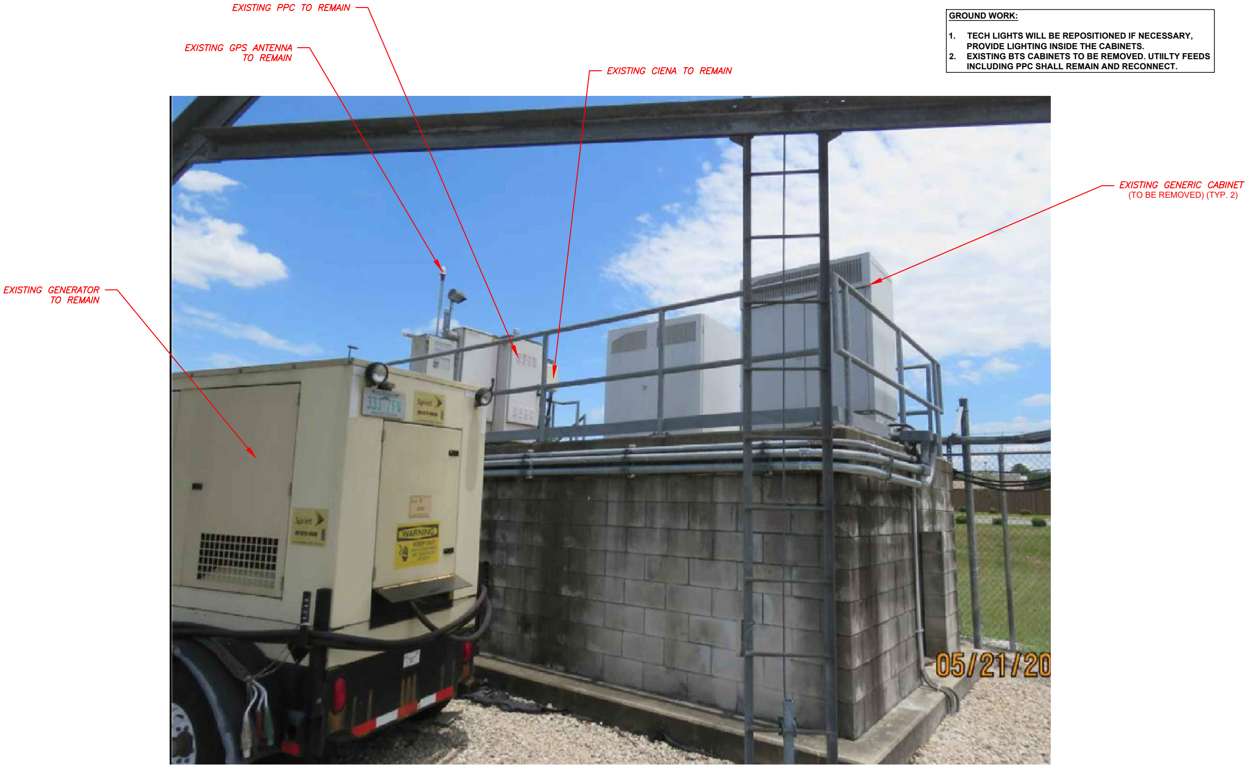
1 EXISTING GROUND EQUIPMENT
