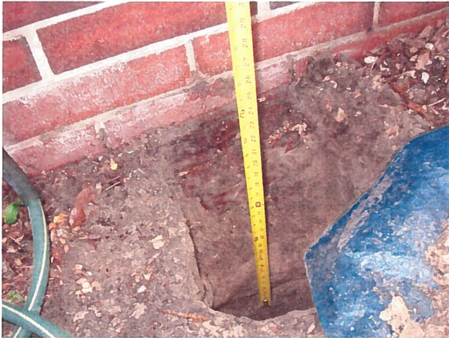
11. Test pit one (TP-1), located near the center of the east wall (see site plan), revealed a foundation embedded approximately 18 inches below ground surface.
