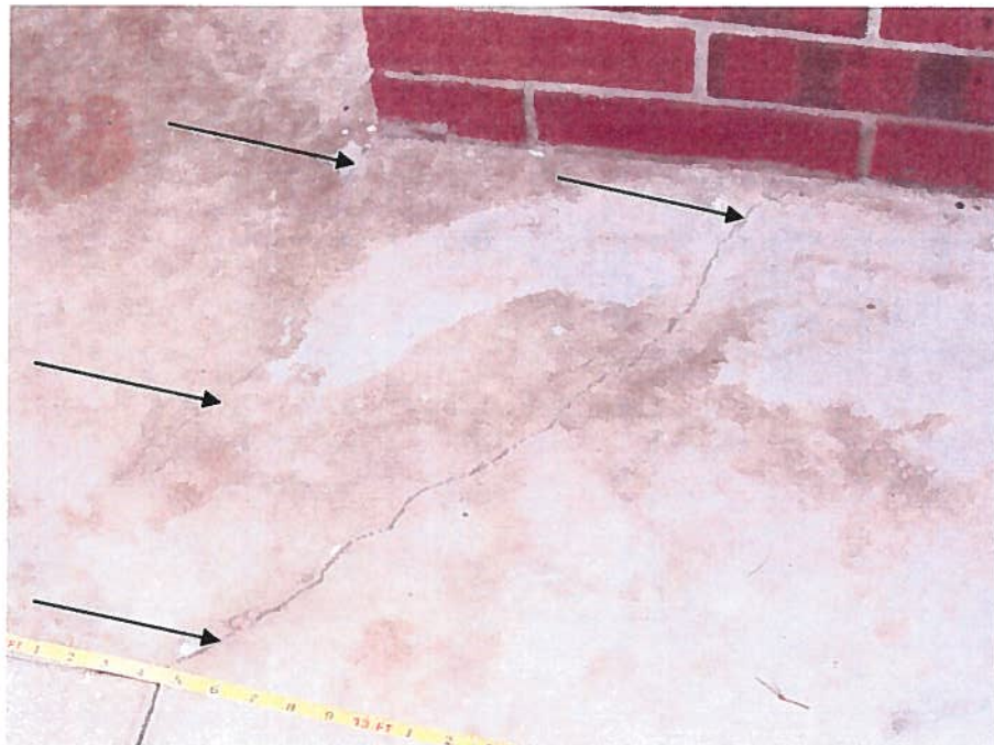
10. Crack in front patio slab, southwest corner
