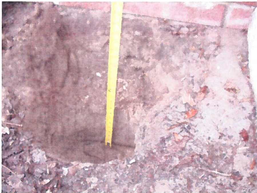
12. Test pit two (TP-2), located near the center of the west wall (see site plan), revealed a foundation embedded approximately 18.5 inches below ground surface.
