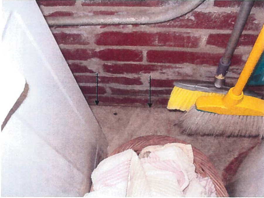
7. Separation crack between floor slab and wall, west side of utility room
