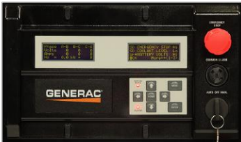
Digital H Control Panel- Dual 4x20 Display
