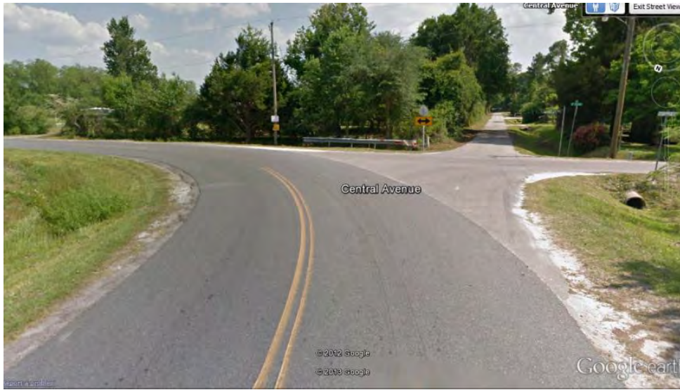
Figure 16. Southbound view of guardrail and exposed culvert end at NE 228th PL/NE 125th Way
